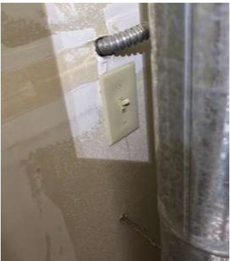
Service shut off switch
